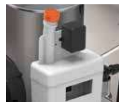
Water tank with anti-scale device
